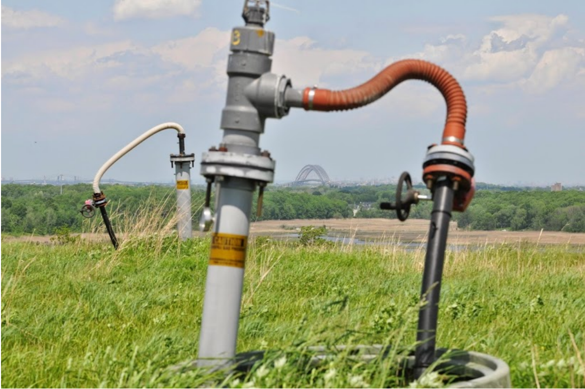
Figure 42. Methane Pumps at Fresh Kills. Source: Google+ non-copyrighted image: https://plus.google.com/photos/at/110251794531052310408?hl=en-US .
